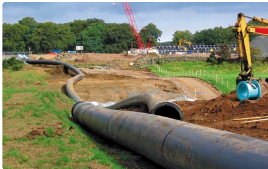
Fig 5: Installation of two PE 100 pipe sections made from Hostalen CRP 100 black in the vicinity of Bankell
