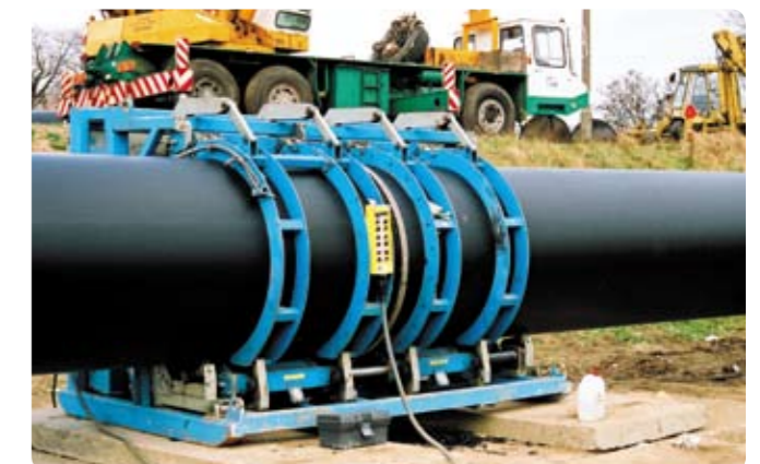
Fig. 3: Hot tool butt welding machine by welding contractor, A.G. Wilson, with PE 100 pipe lengths made from Hostalen CRP 100 black
