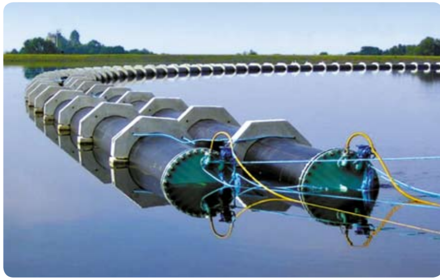
Fig 4: Twin Marine Pipelines DN 1100 made from Hostalen CRP 100 black (PE 100) prepared to be placed in the Craigmaddie Reservoir
